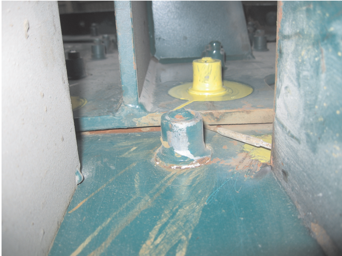
Fig. 3. Lasting deformation of the support
