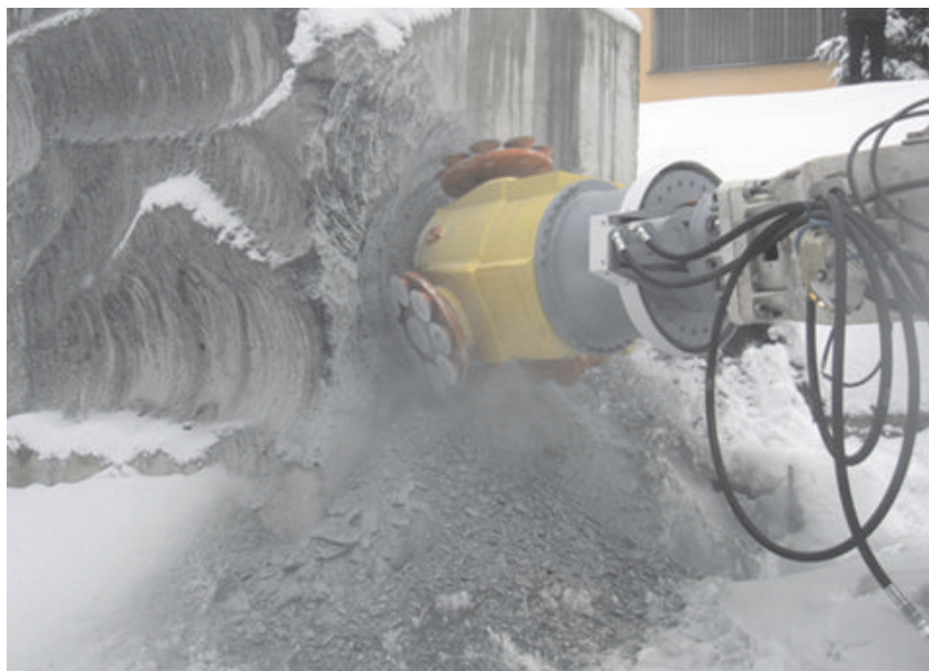
Fig. 13. A view of the KR 150 roadheader with the new solution of a head with asymmetrical disc tools of complex motion trajectory during one of the field tests for the most favourable selection of direction and number of rotations of the head body and plates with tools
