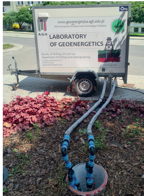
Fig. 1. TRT Equipment (photo Geoenergetics Lab team)
