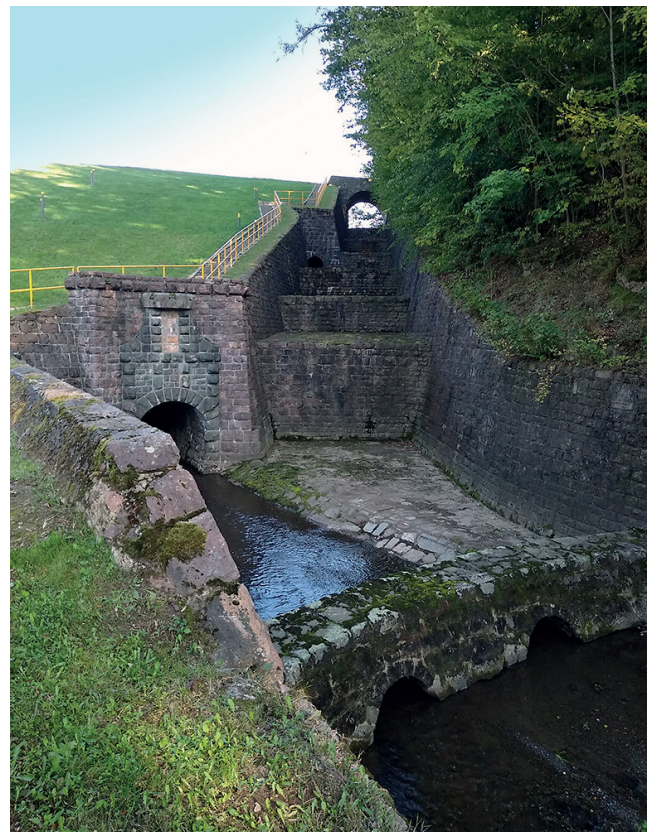
Fig. 7. The dam on the dry flood reservoir in the Świerzawa town. Photo P. Słomski
