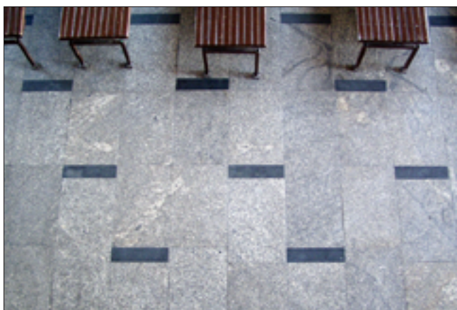
Fig. 9. General view of flooring slabs of Strzegom granite (grey), quartz diorite and monzodiorite of Przedborowa (black) inside the former bus station „PKS Wieluń”, photo A. Śpiewak
