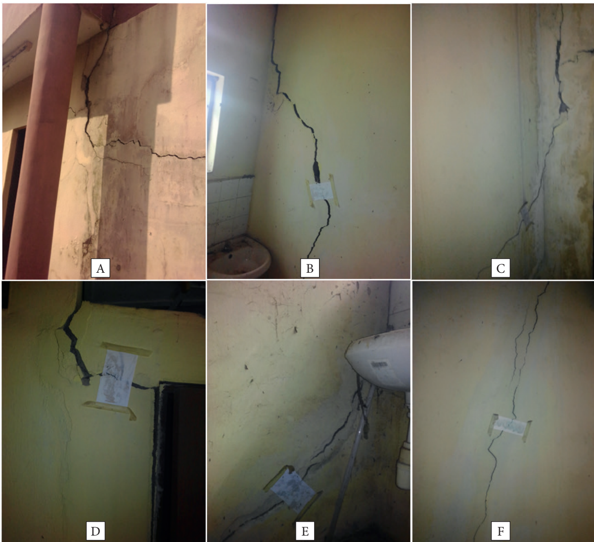
Fig. 1. Pictures of stress induced cracks in adjacent building located about 70 m southeast of the proposed construction site
